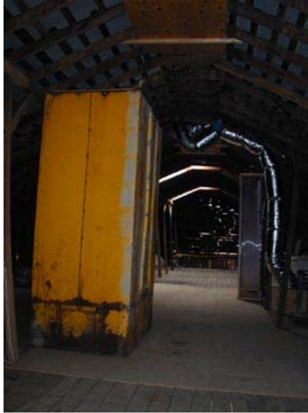
Figure 9. The vacuum equipment for the picker, in the upstairs loft of the barn.
