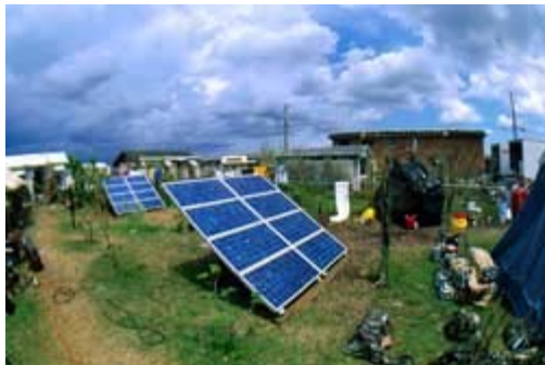
Photovoltaic arrays may serve as temporary, stand-alone power sources in a disaster area. (Photo: Robin Flynn)
